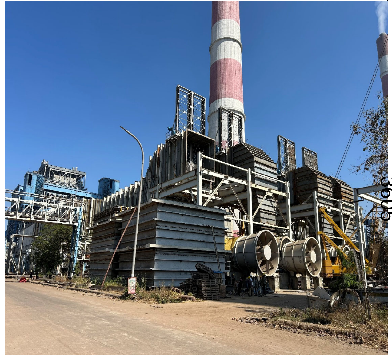
Duct U#5 – Booster Fan Inlet duct completed with exsisting plant duct connection
