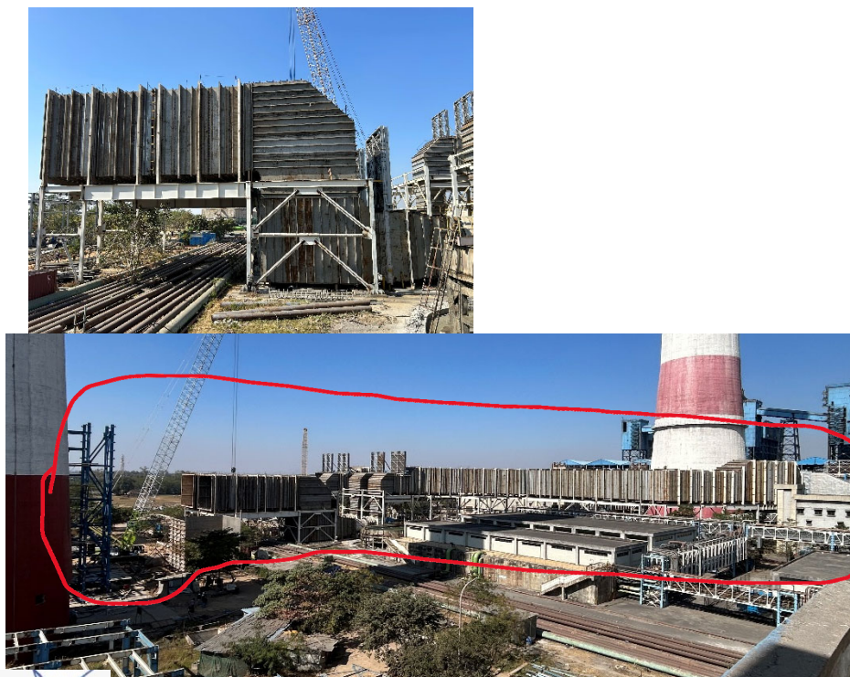
Duct U#4 – Booster Fan Inlet Side duct almost ready, out let duct erection started
